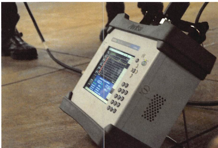
Image 17 - Transit Wireless Test equipment
