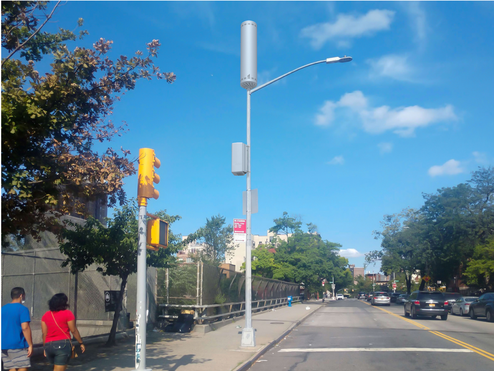
Standard FS Streetlight
